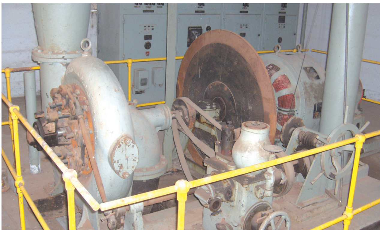
Interior of the old hydroelectric station at the Hartbeespoort Dam in South Africa.
