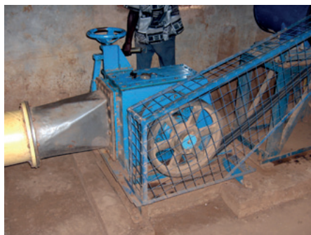
Tungu-Kabiri's 18 kW crossflow turbine ▼
