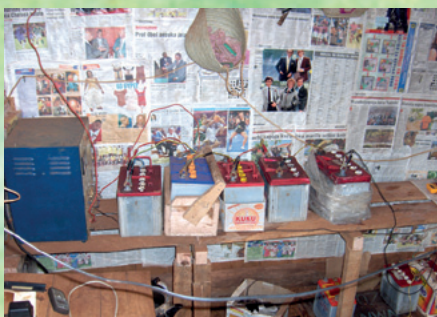
Car Battery charging, to provide domestic lighting ▼
