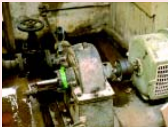
The pelton turbine in the Svinurayi powerhouse.
